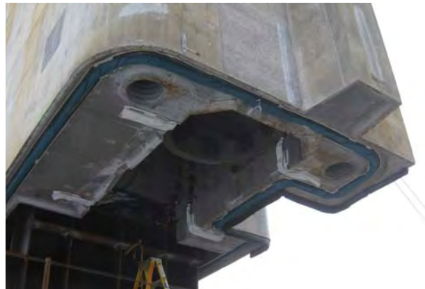
Condensed Grout Bag Base Seals Under a Pier Shell Caisson (Blue)
