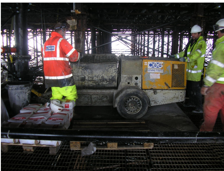
Automated Pumping Plant
