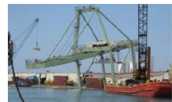
Figure 11. Collapsed Container Berth
