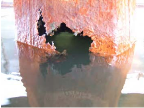
Figure 29: Holed Pile Due To ALWC
