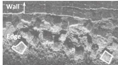
Figure 15 Plan Survey Of Edge Scour To Precast Block Toe Protection (Tomlinson et al , 2003)
