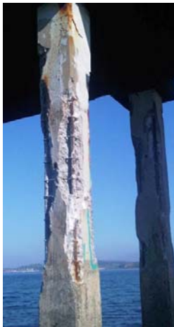
Fig. 7 - Damaged R.C. Pile, Hunterston
