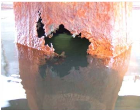
Fig. 1 – ALWC Damage. Dublin Jetty
